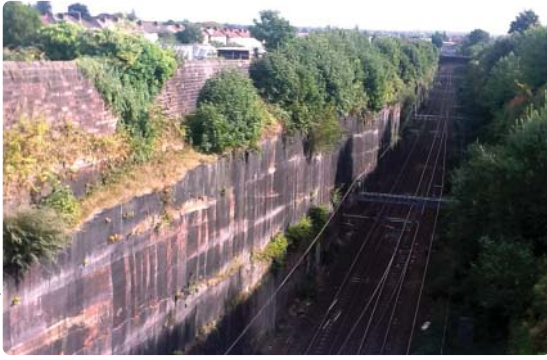
Olive Mount cutting—excavated by hand, with a little help from gunpowder; subsequently widened and recently electrified
